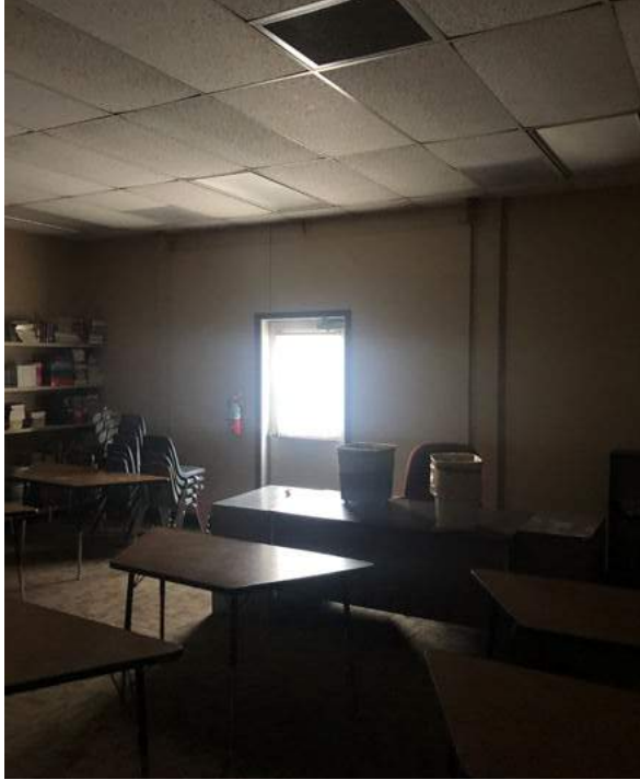
No insulation in Room 301, used to have a garage door.
