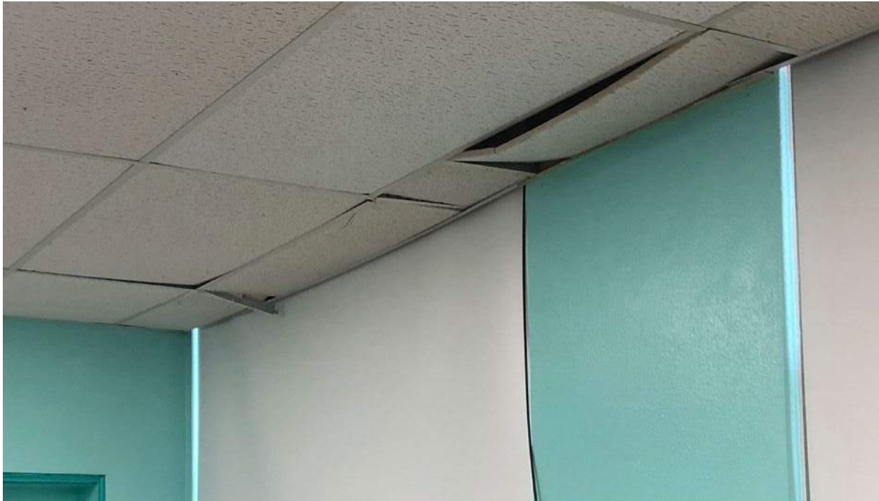
Ceiling tiles and grid are sagging and falling apart.
