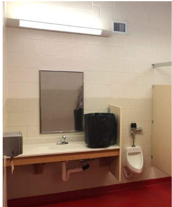
Sink in boy's locker room is not handicap accessible.
