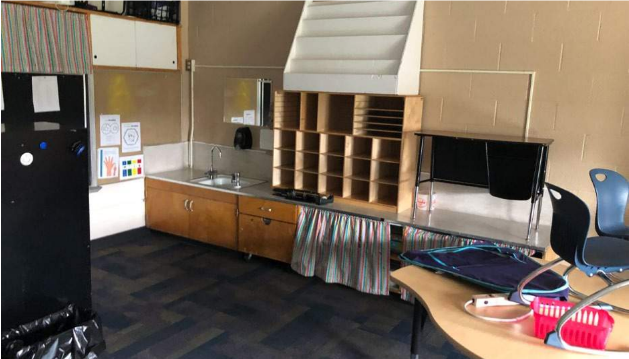
Casework is aged in older classrooms and sinks do not meet handicap accessibility.
