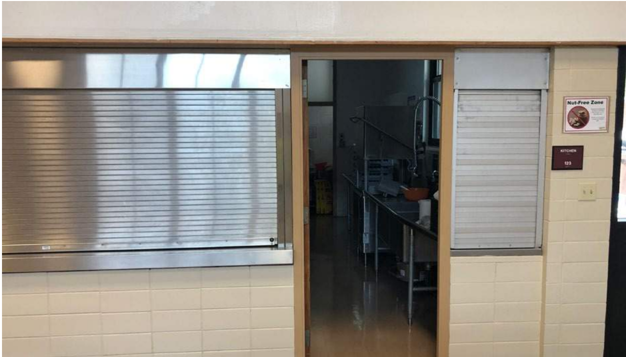
Door to kitchen does not meet push/pull clearance.
