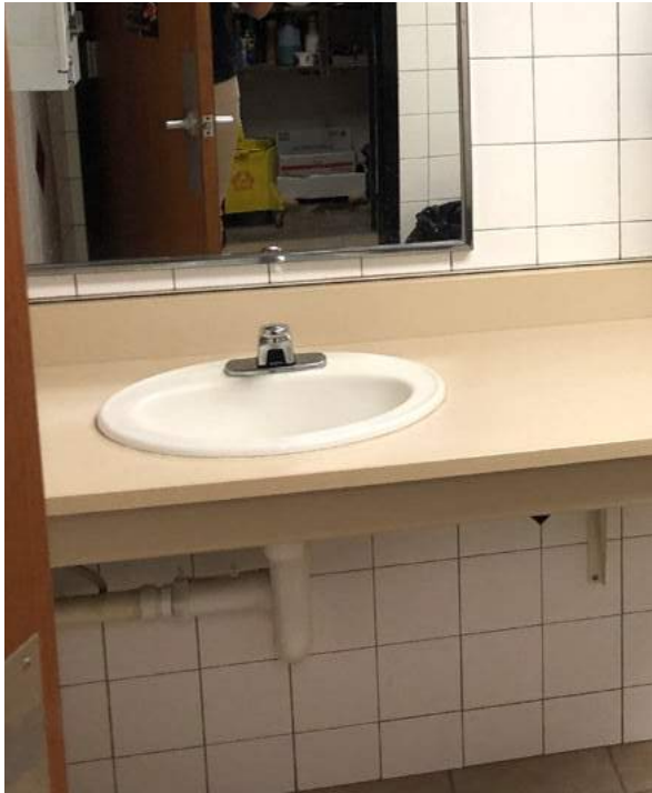
Sink is not handicap accessible in women's bathroom.
