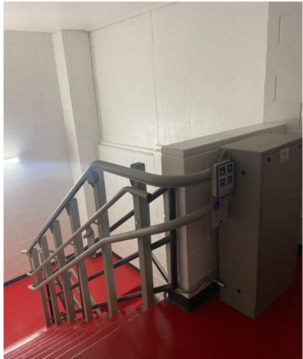
Hand and guard rails on stairs are not to code.
