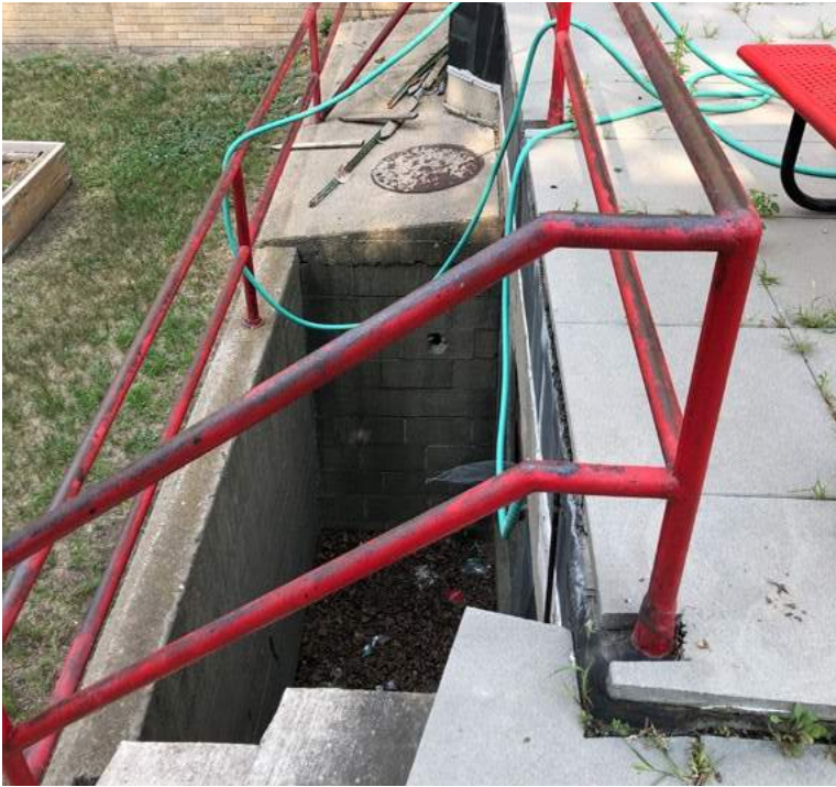
Handrails on steps in courtyard are not to code.
