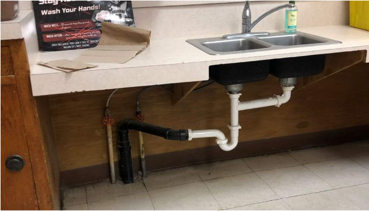
Exposed pipes underneath means this sink is not handicap accessible.
