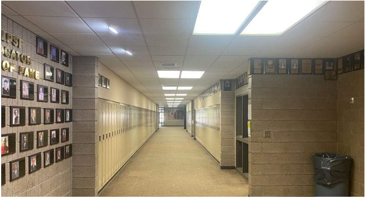
Ceiling tiles are in adequate shape, but the grids are yellow.
