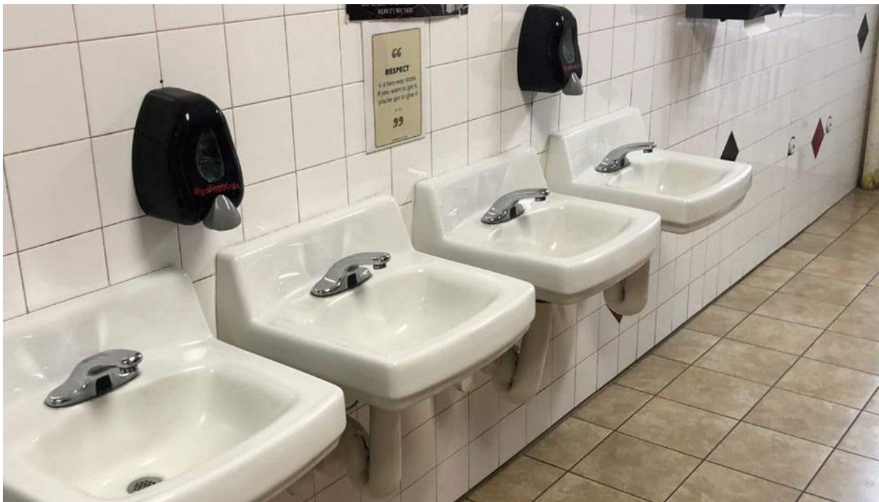
Sinks do not meet handicap accessibility. They are too low and have exposed piping that does not meet required clearances.
