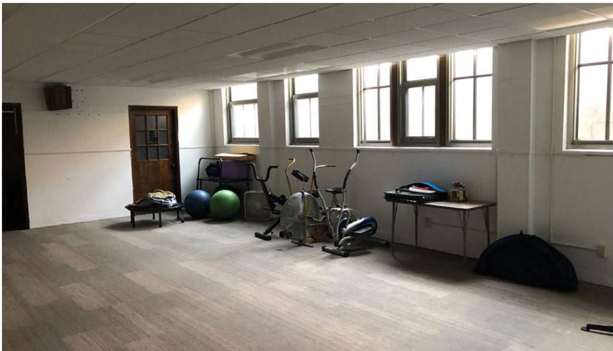
Basement windows in classrooms are not up to code. Egress windows are too high, and do not allow to adequate egress into the courtyard.
