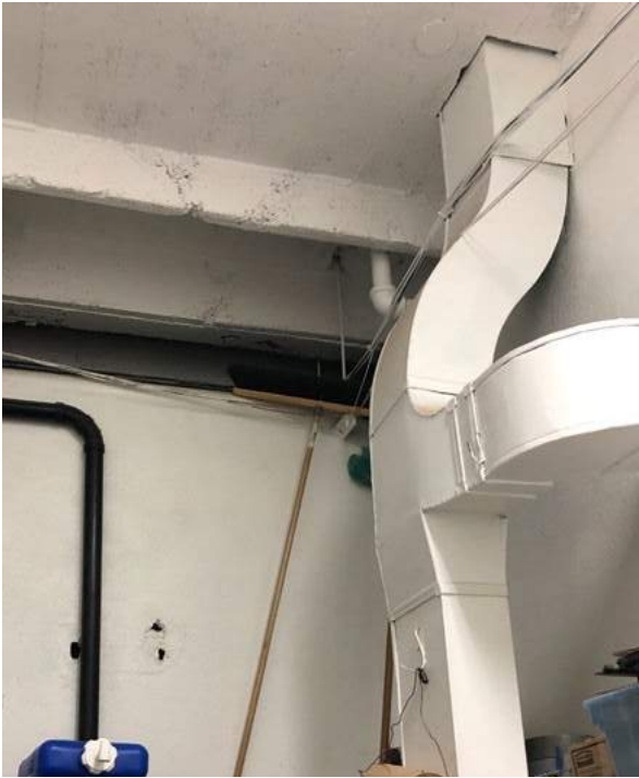
Exposed wiring in custodial closet.
