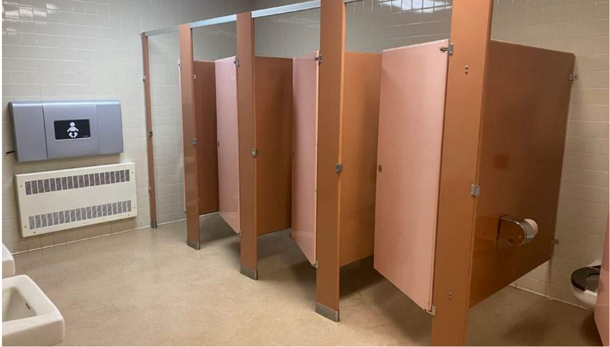
Toilet partitions need a refresh in the women's restroom.
