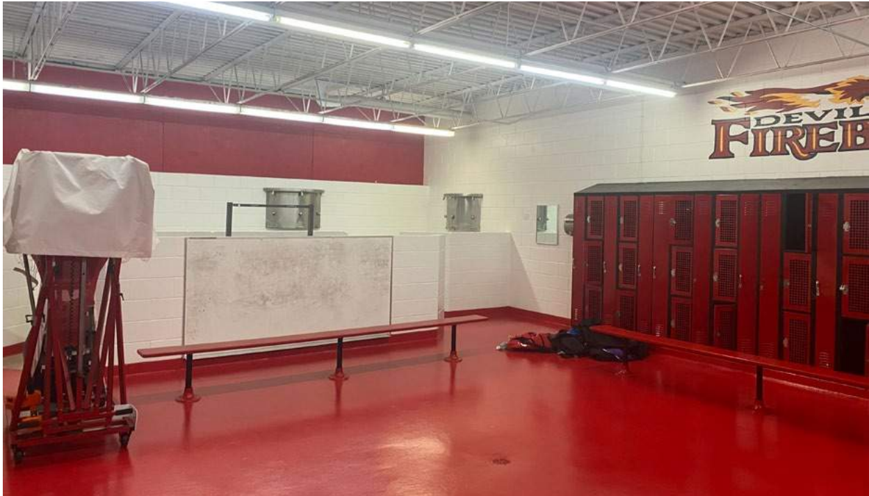
There are no handicap accessible shower stalls, sinks, or drinking fountains in the locker rooms.
