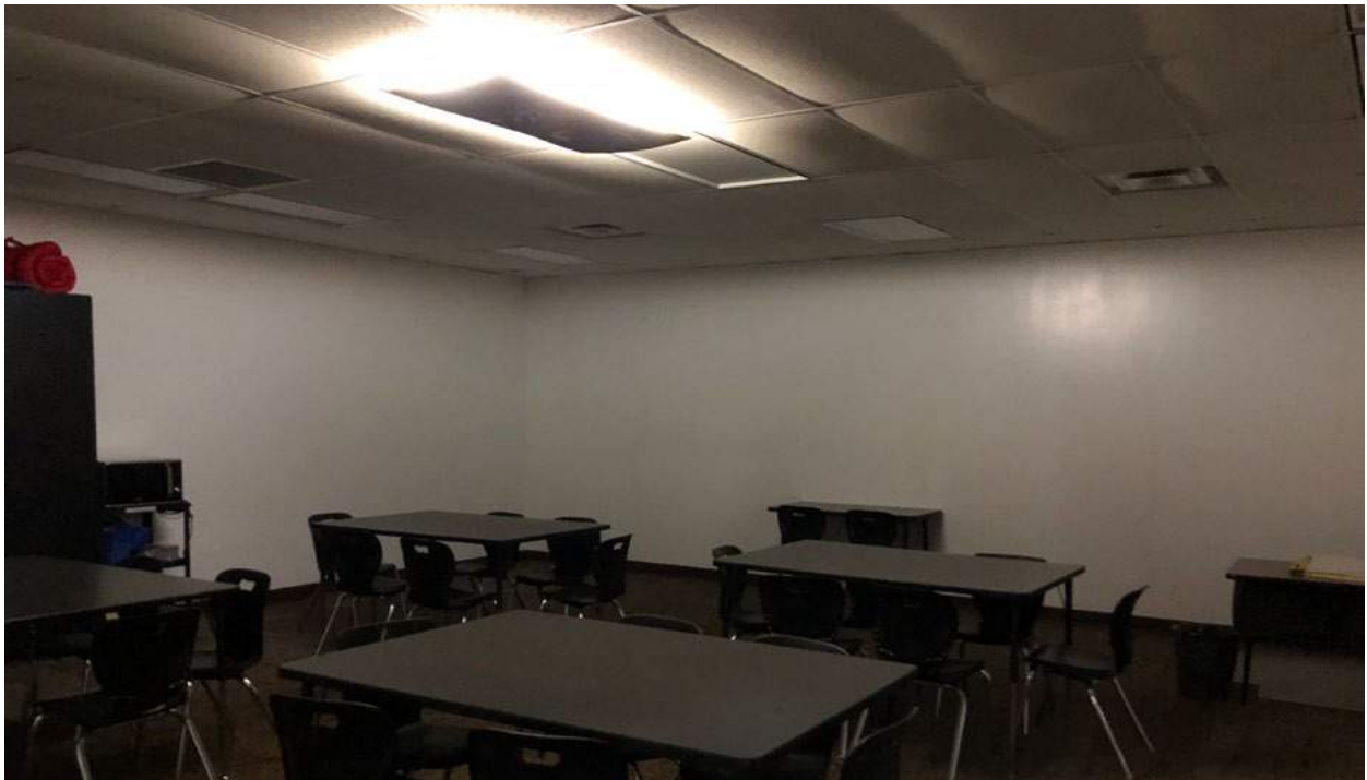
Ceiling tile is in bad shape throughout all the classrooms.
