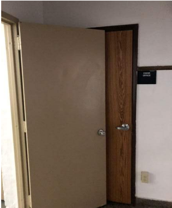
Doors are overlapping.
