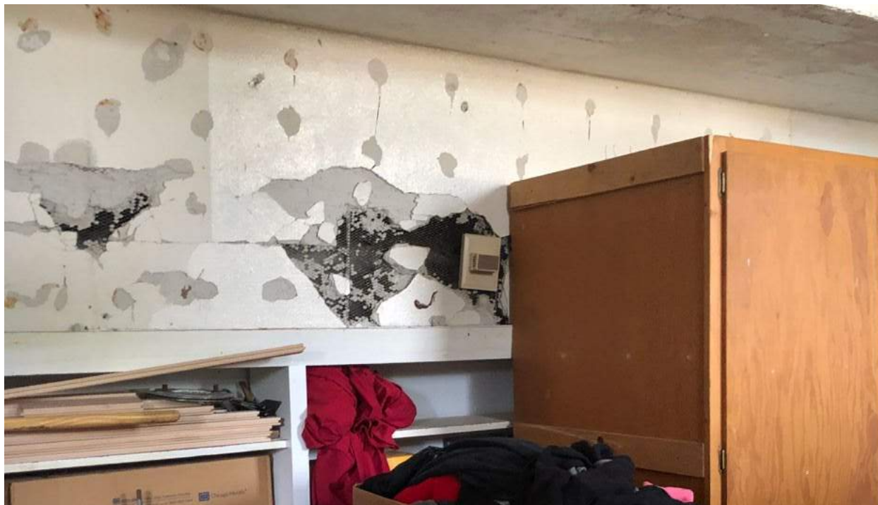
Wall has various damage marks.
