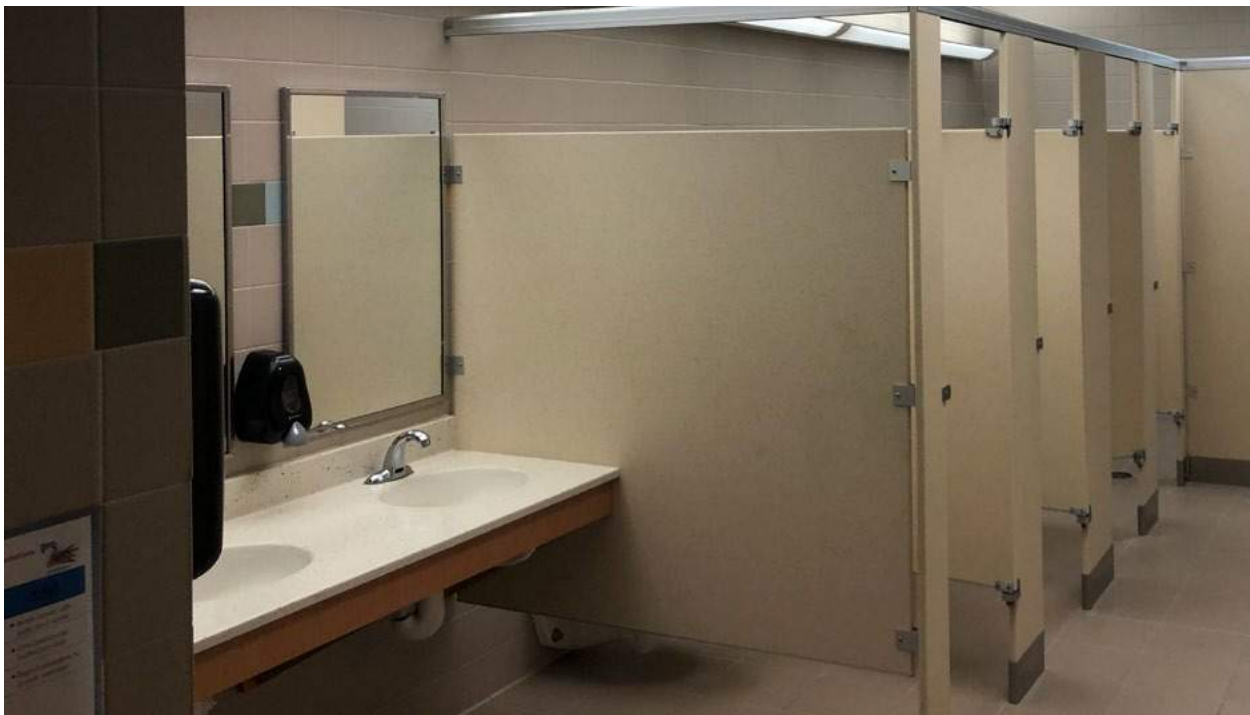
Sinks are not handicap accessible in both boy's and girl's restrooms.
