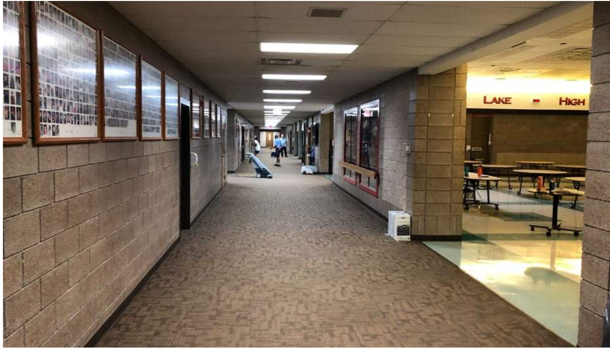
No sprinkler system.
