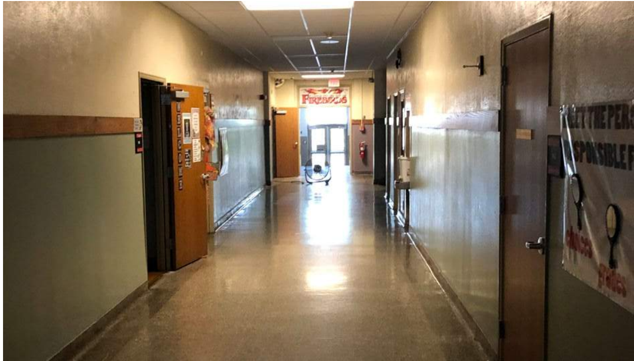
No sprinkler system throughout entire building.
