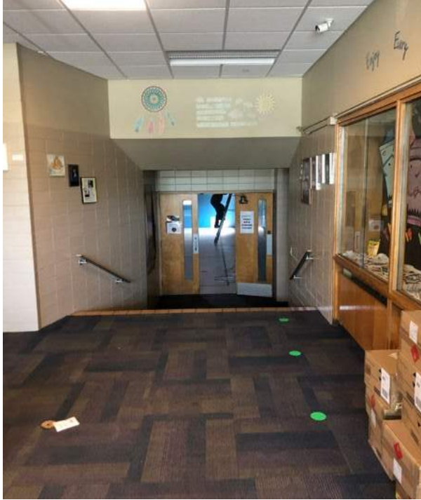
Gymnasium and associated spaces are not handicap accessible and lack adequate handrail and guardrails.
