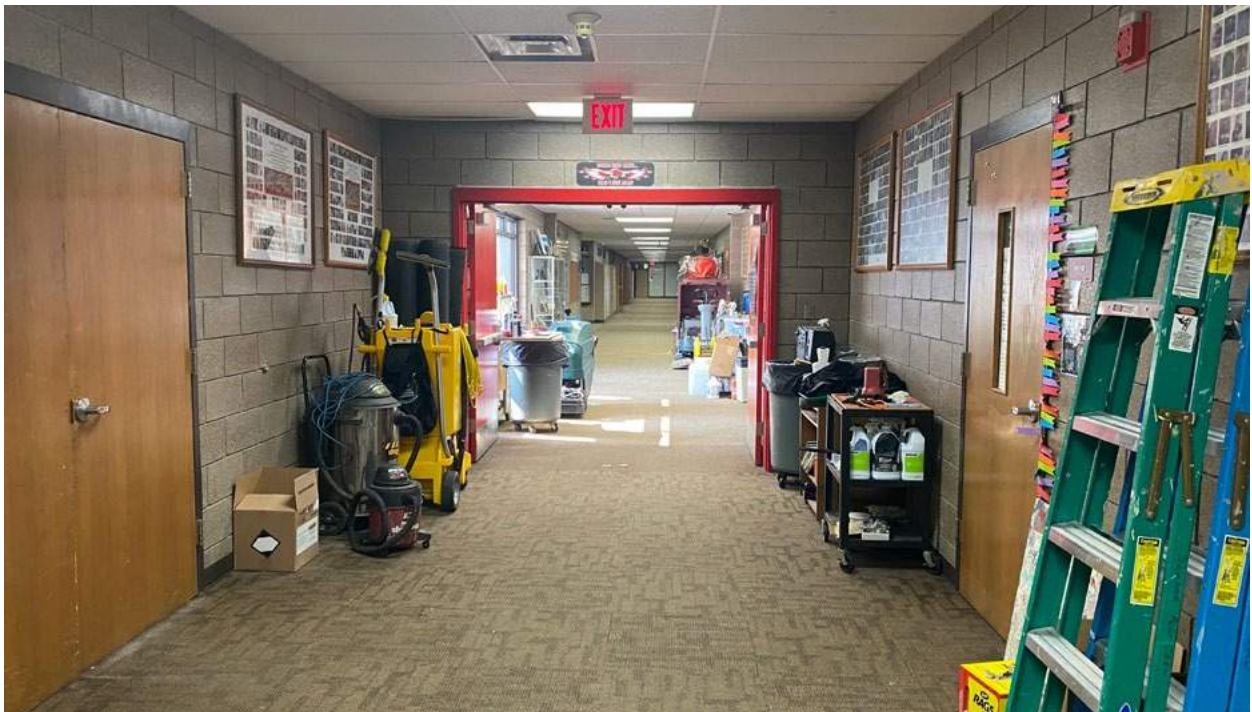
Corridor doors and frames are not fire rated and are aged. Panics on some doors are aged.
