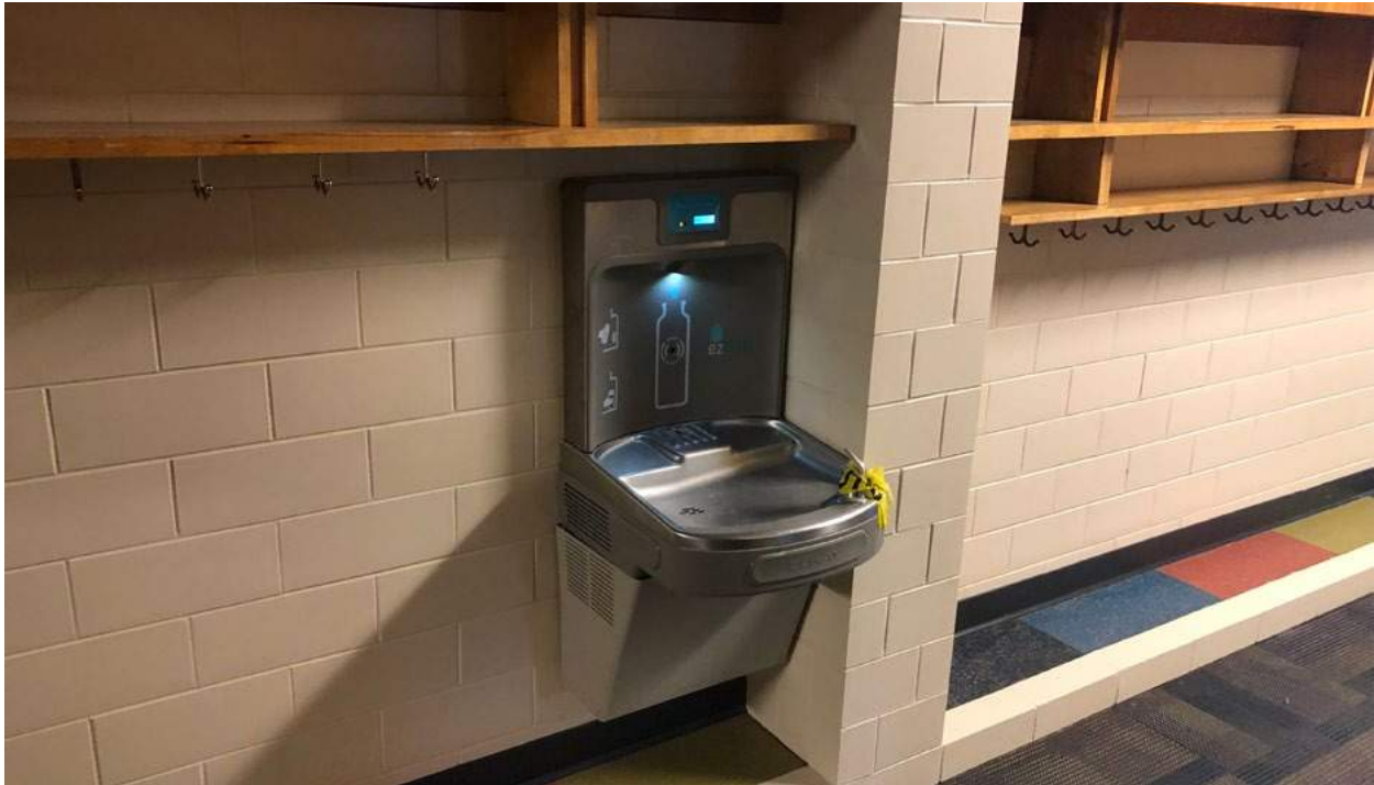
Drinking fountain in corridor is not code compliant.
