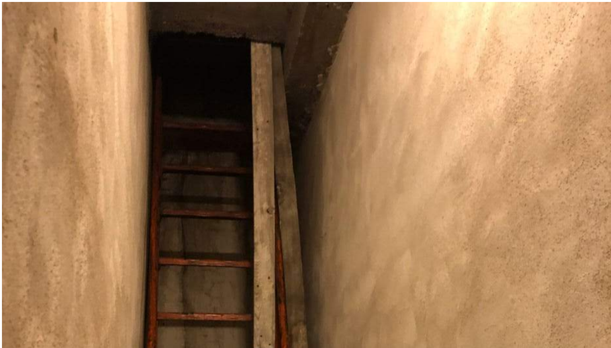
There is no door to the roof access.
