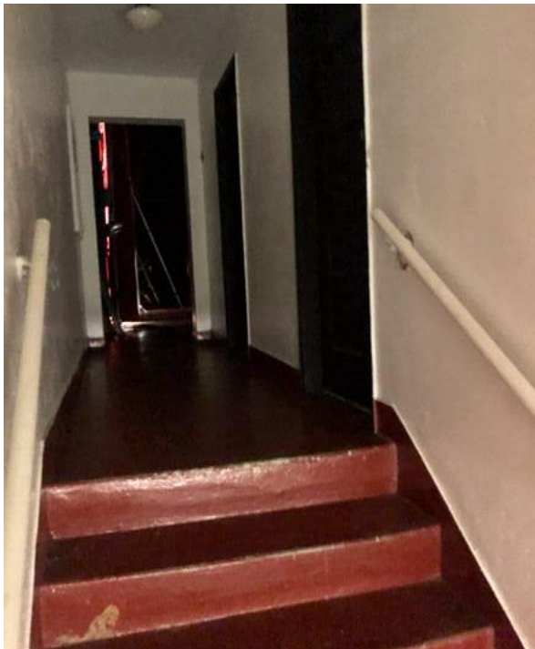
Stage is not handicap accessible, only has stairs.
