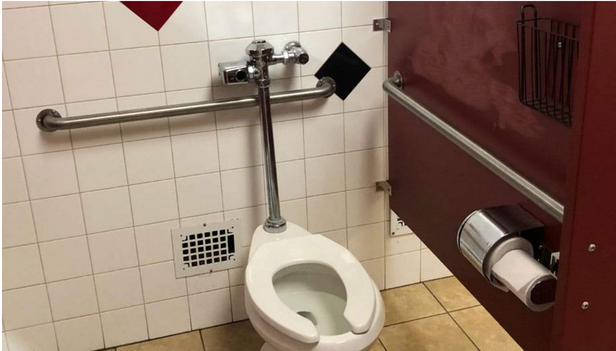
There is no vertical grab bar in the ADA stall in boy's bathroom.
