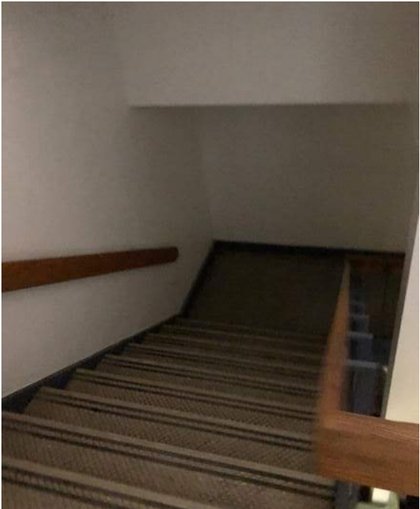
Stairs to basement do not meet code requirements; missing adequate handrail and guardrails.
