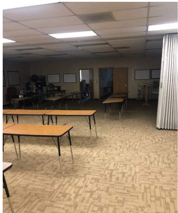
Alternative HS classrooms have no acoustic control and are considered intervening spaces, and are not code compliant.
