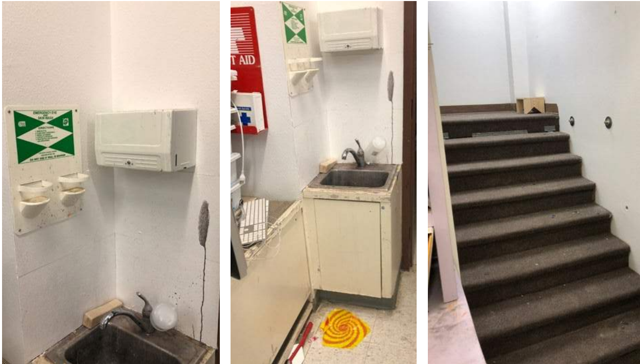
Room 104 stairs, sinks, and emergency eye wash station not up to code or handicap accessibility requirements.
