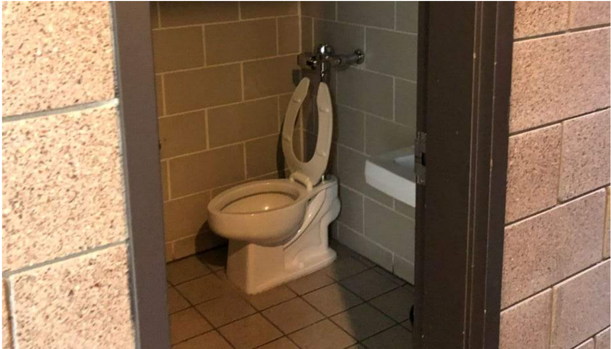
The single restroom on the second floor is not handicap accessible.
