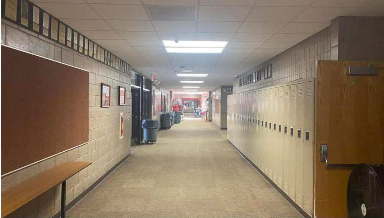
No sprinkler system.
