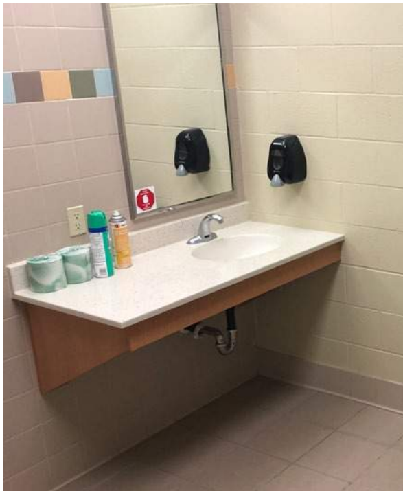
Sink in family restroom is not handicap accessible.
