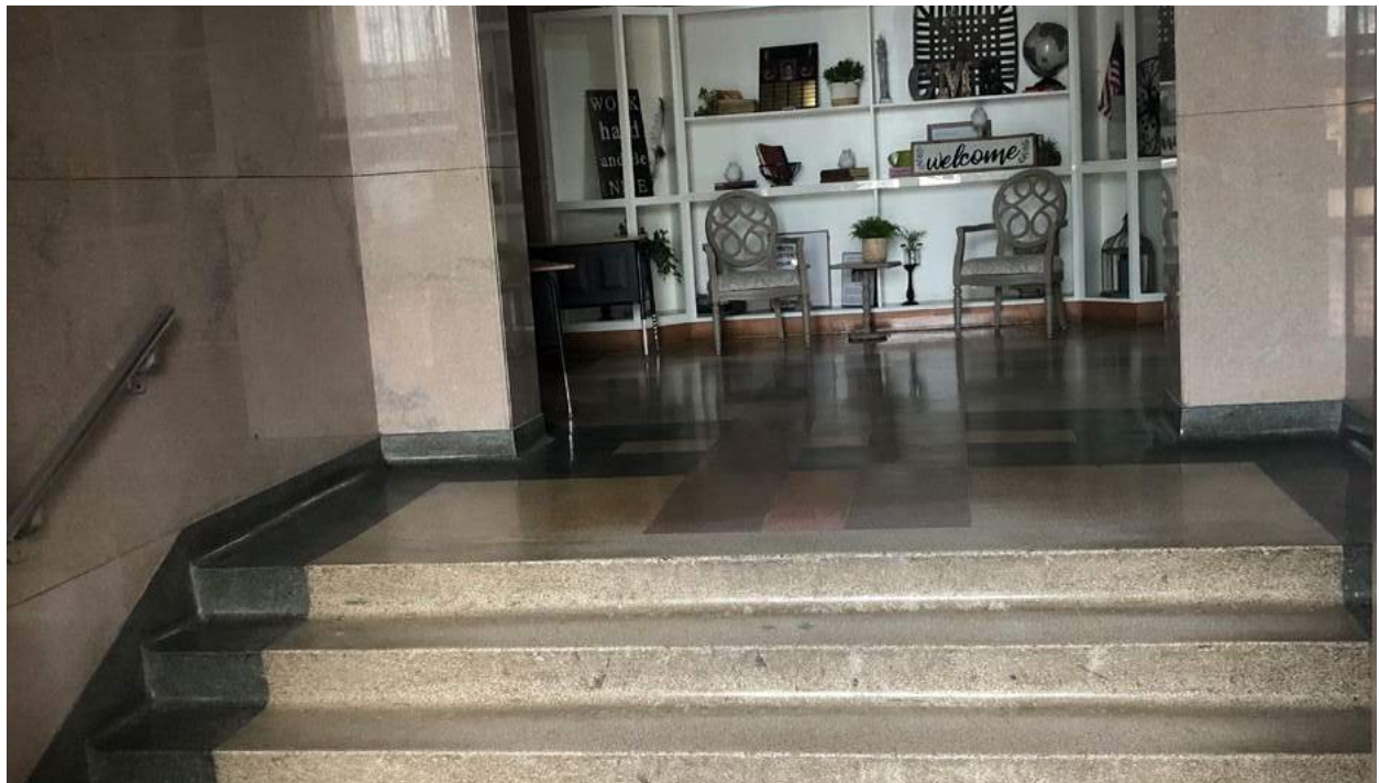
Main entrance not accessible. Handrails not to code. There is no ramp or middle railing.
