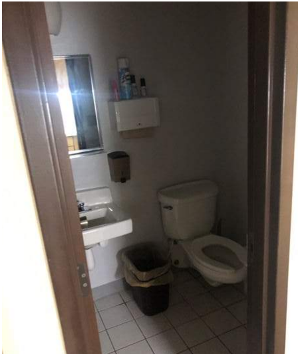
Toilet in staff room restroom is not handicap accessible.
