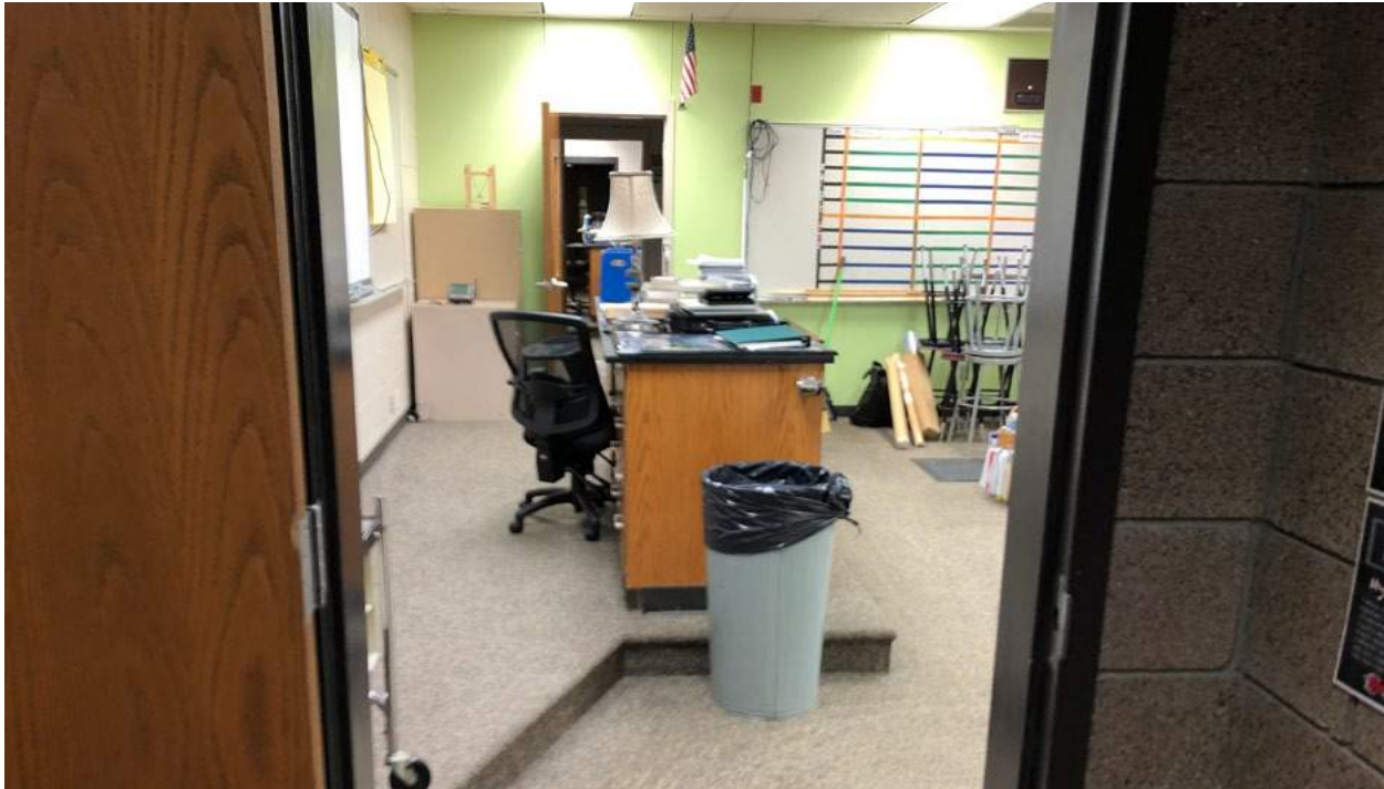
Raised teaching platforms in Science rooms are not accessible.
