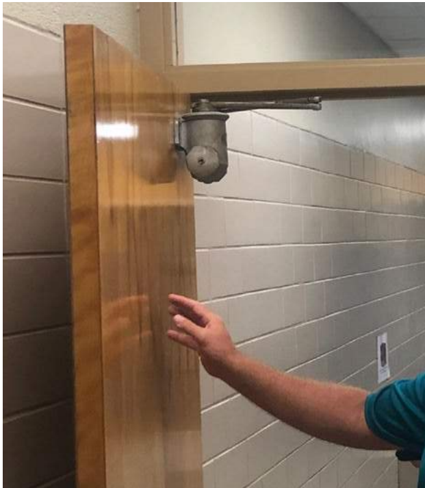
Doors and door hardware are aged.
