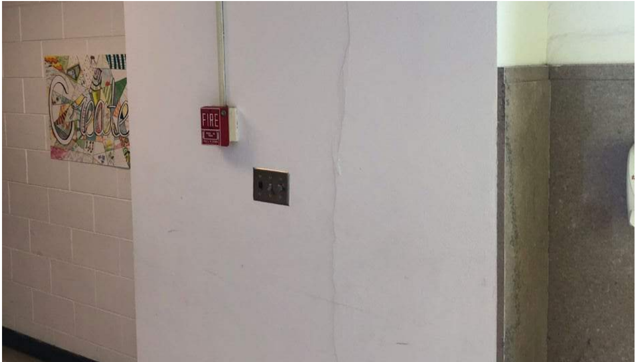
Crack and/or water damage on corridor wall.
