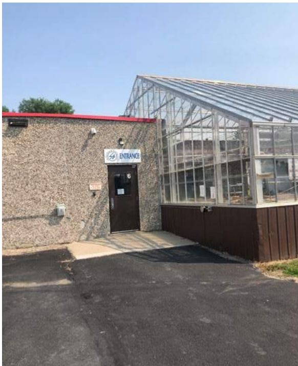
Student entrance is not a secure entry and lacks an interior vestibule.
