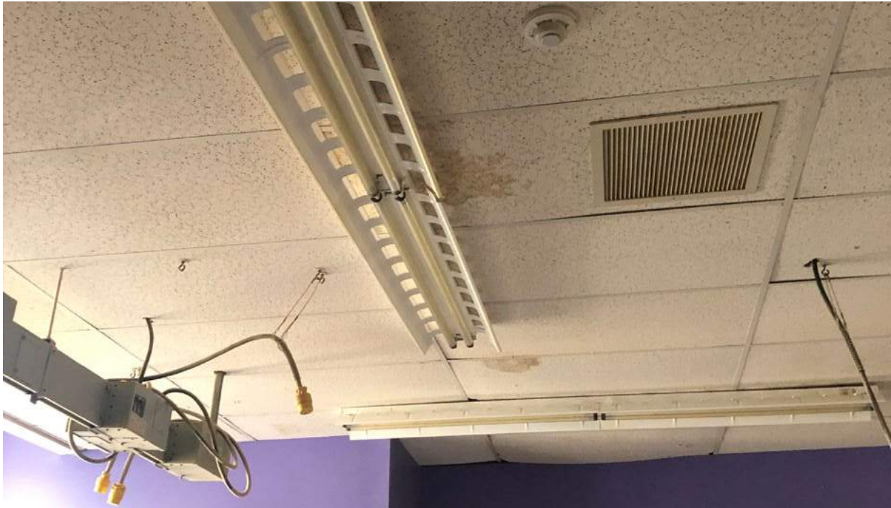
Room 104 Shop: Ceiling tiles in very bad shape. Water leaks on the ceiling.
