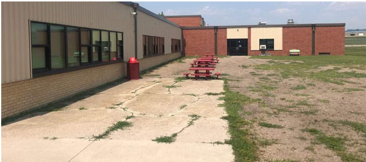
Cracked and settling concrete.
