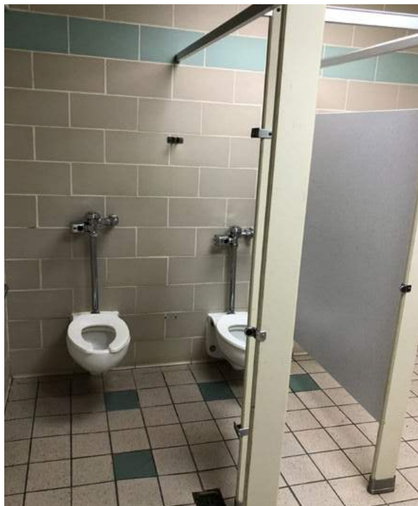
Missing stall doors in men's restroom.
