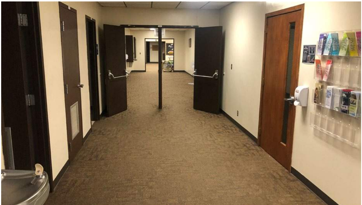
Doors and frames in corridor are not all fire rated.
