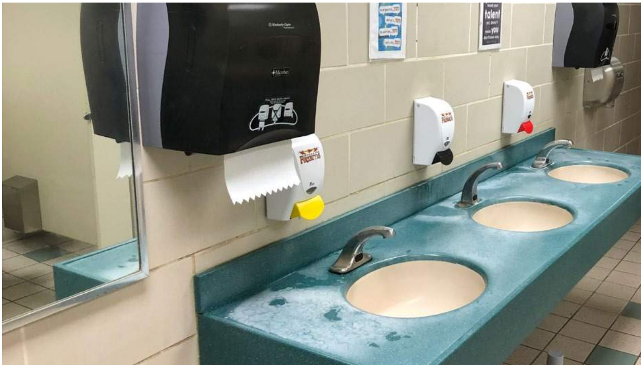
Sinks, soap dispensers, and paper towel holders in men's and women's restrooms are not handicap accessible due to reach ranges.
