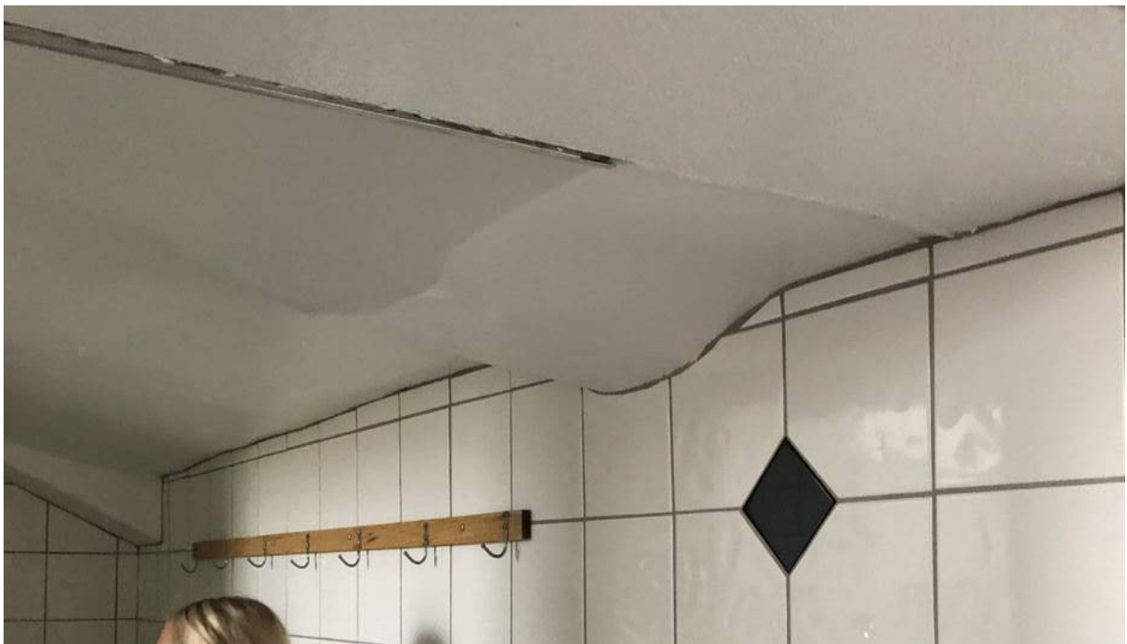
Ceiling caving in boy's locker room.
