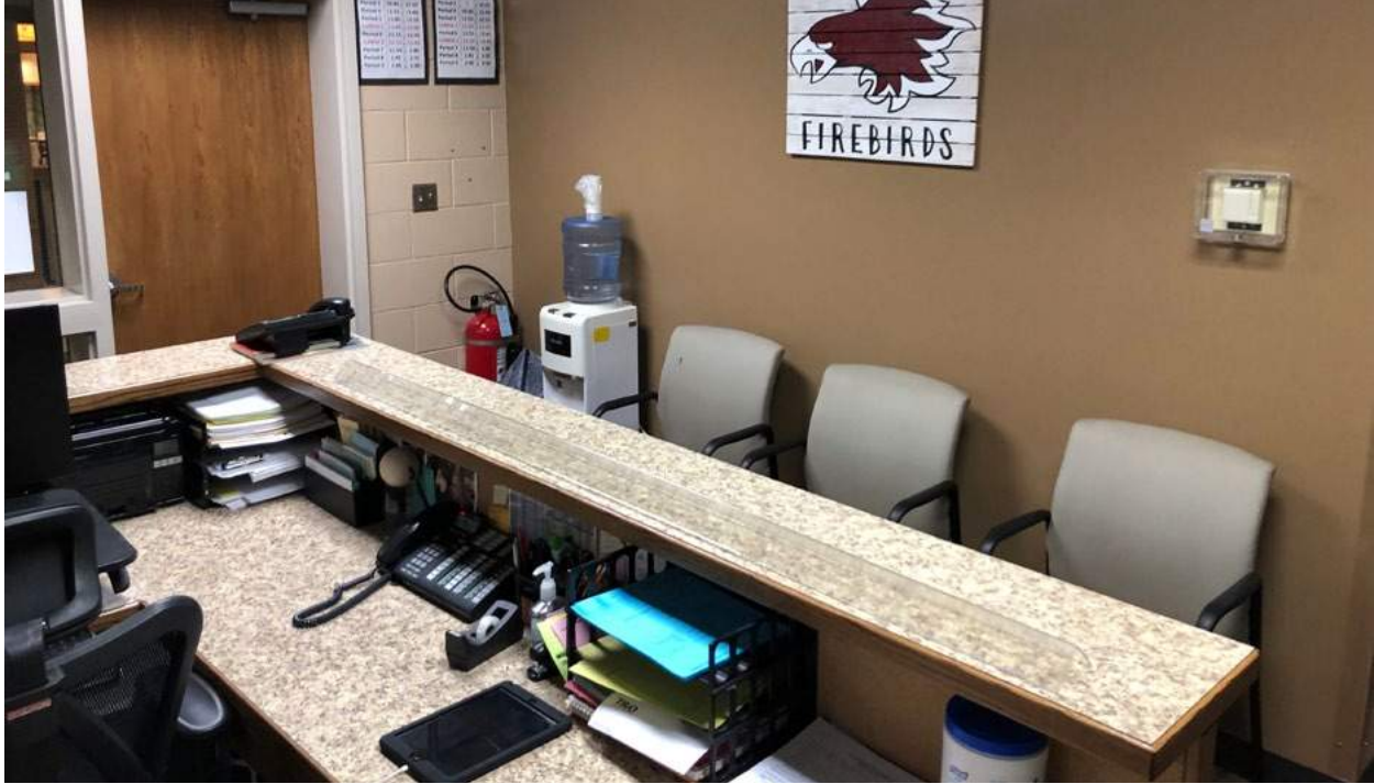
Main office does not have a handicap accessible reception desk and there is a lack of waiting space.
