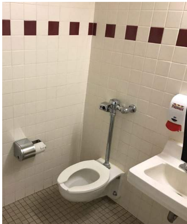
Staff restrooms are not handicap accessible and are missing grab bars.
