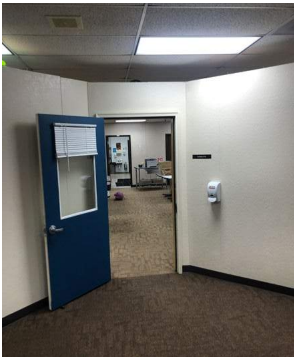
Walls for culinary arts classroom don't meet the ceiling.
