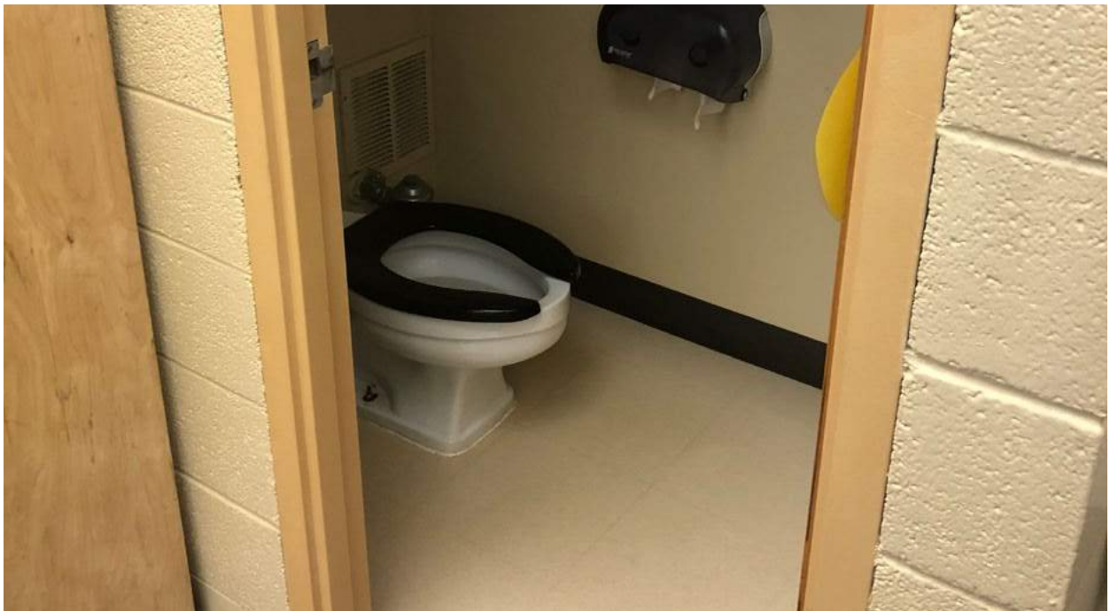
Restrooms in classrooms are very small and do not meet maneuverability and clearance requirements.
