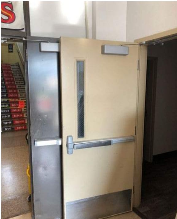
Vestibule and corridor doors overlap.
