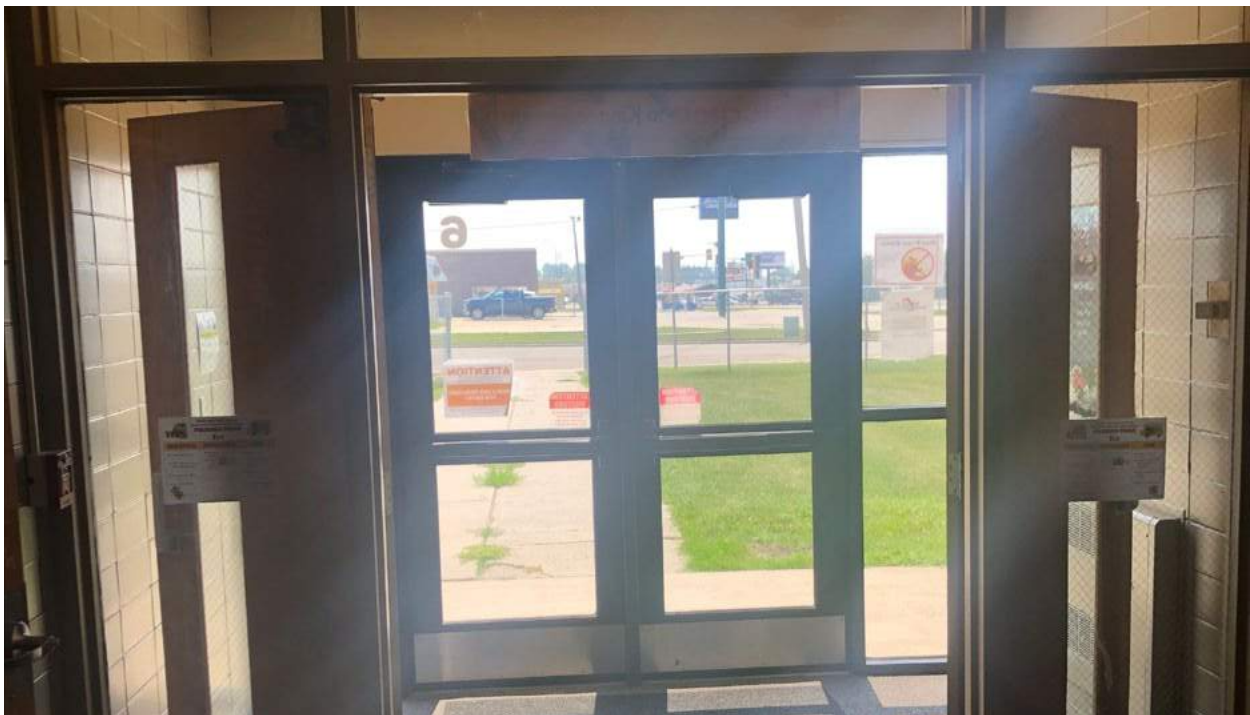
Interior vestibule doors do not have a closer.
