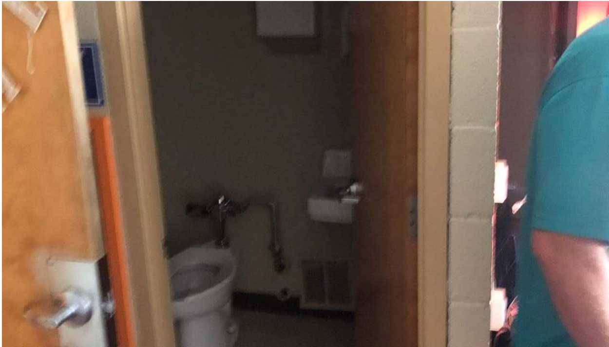
Restroom in Resource Room and Staff Lounge are not handicap accessible.
