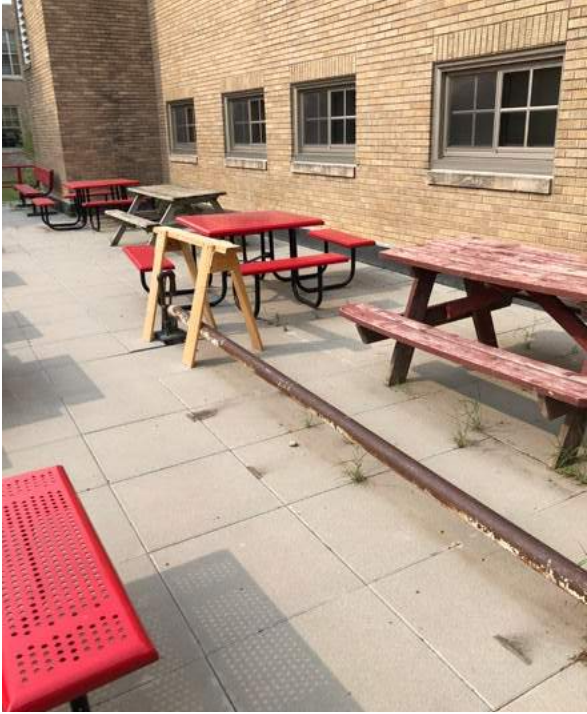
Exposed piping in the courtyard area.
