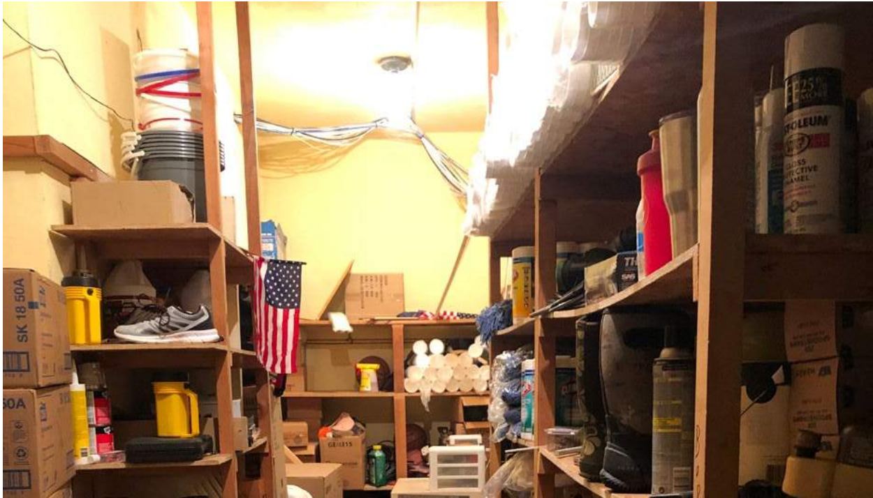
Exposed electrical wiring in storage area.
