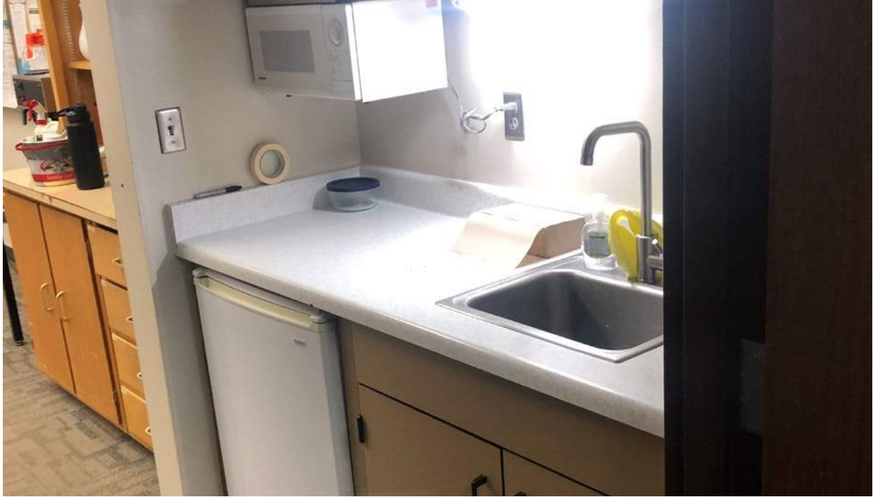
Sink and countertop not handicap accessible in staff room.
