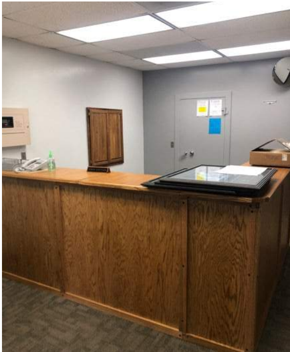
Casework in main office is not handicap accessible.
