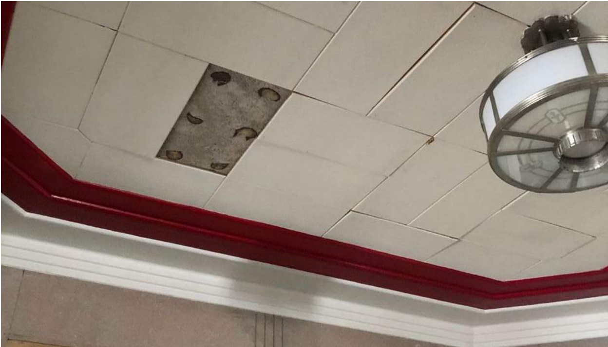
Missing ceiling tiles in main entrance area.
