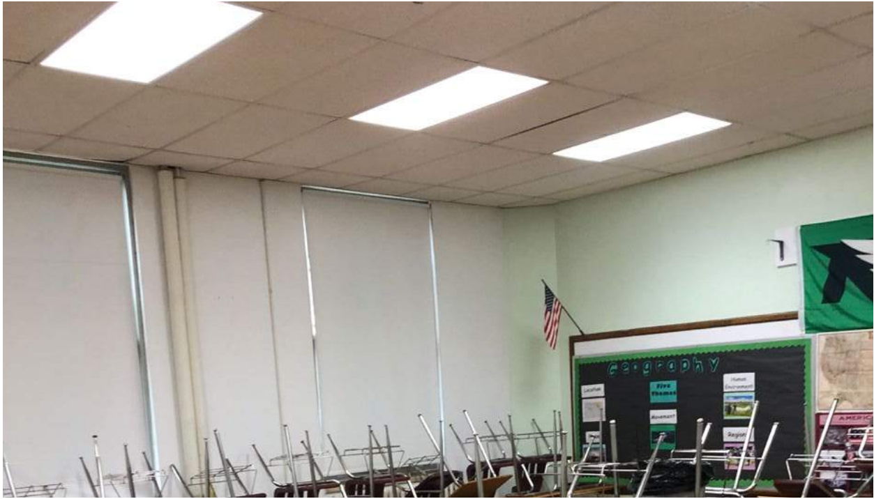
Ceiling tiles are in bad shape throughout the building.
