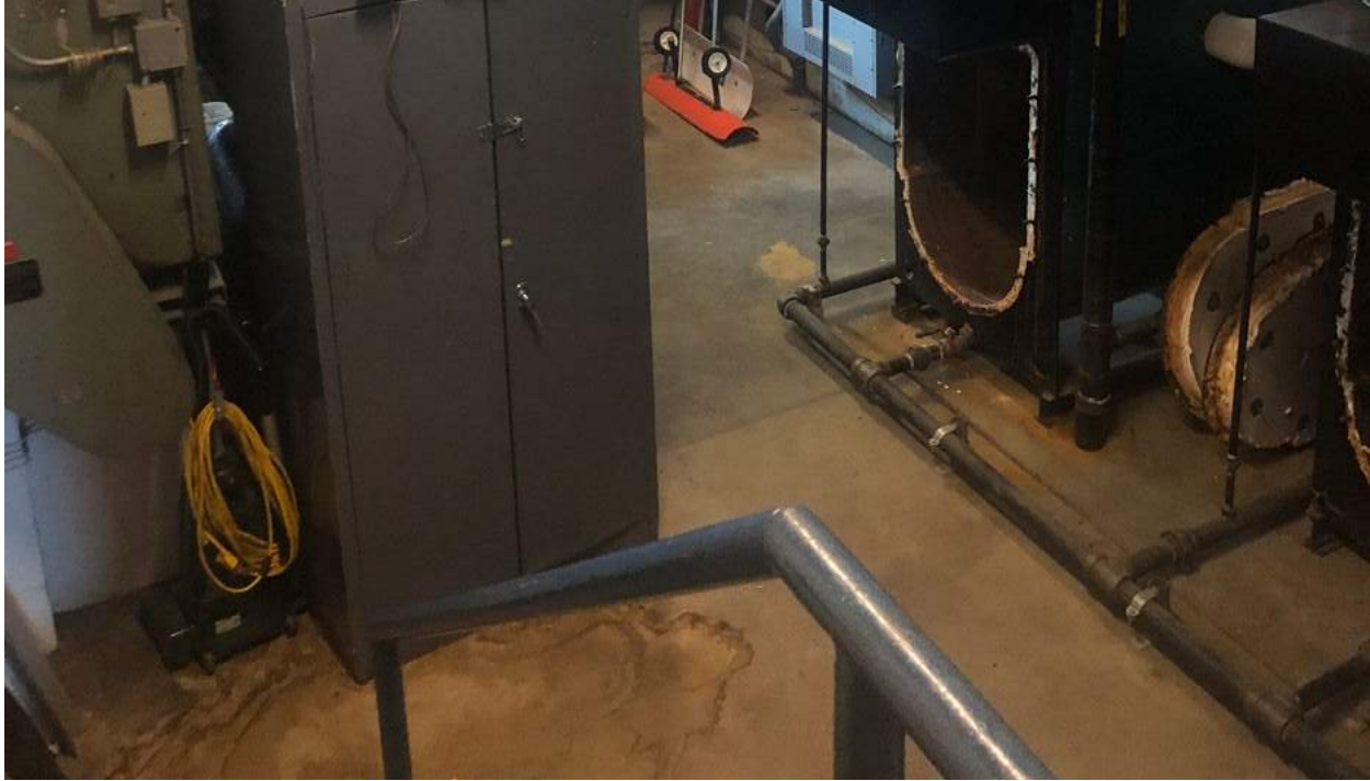
The boiler room is not handicap accessible. Existing stairs are not to code.
