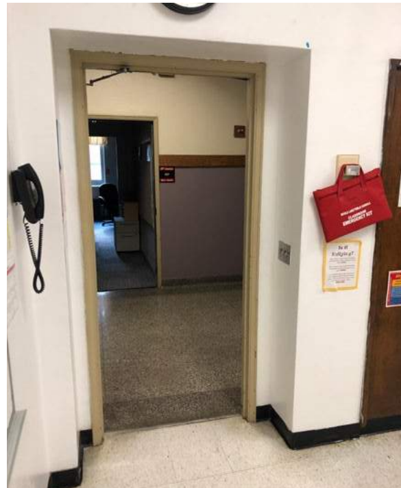
Classroom doors do not all have the minimum push/pull clearances required for handicap accessibility.
